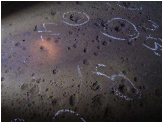
SRB pitting corrosion of tank floor
