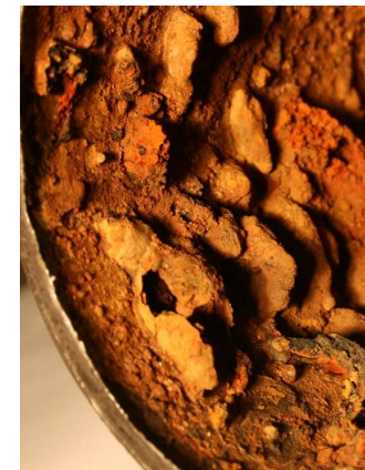
Deposits from long term corrosion
