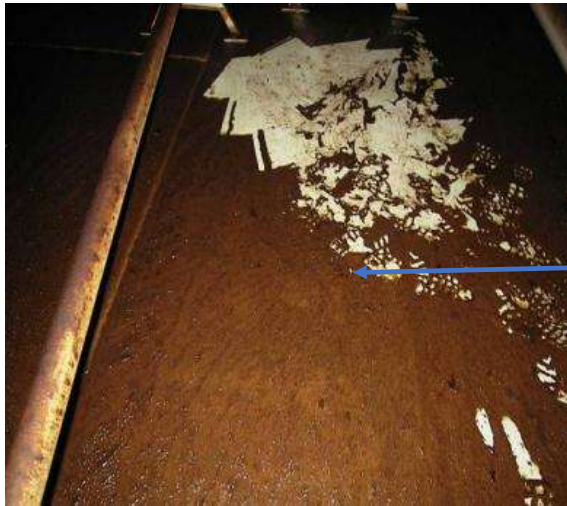
Microbial biofilm in jet fuel storage tank
